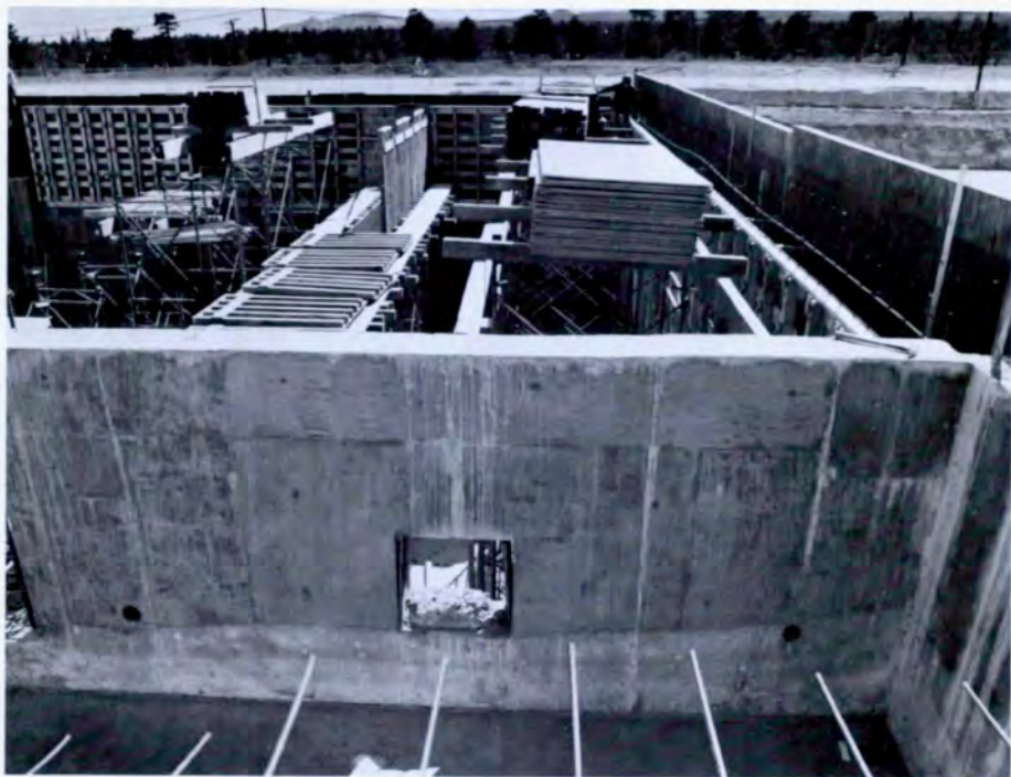
Harold helped convince the AEC of the absolute necessity for a new plutonium research and development facility. Construction started in 1974.
